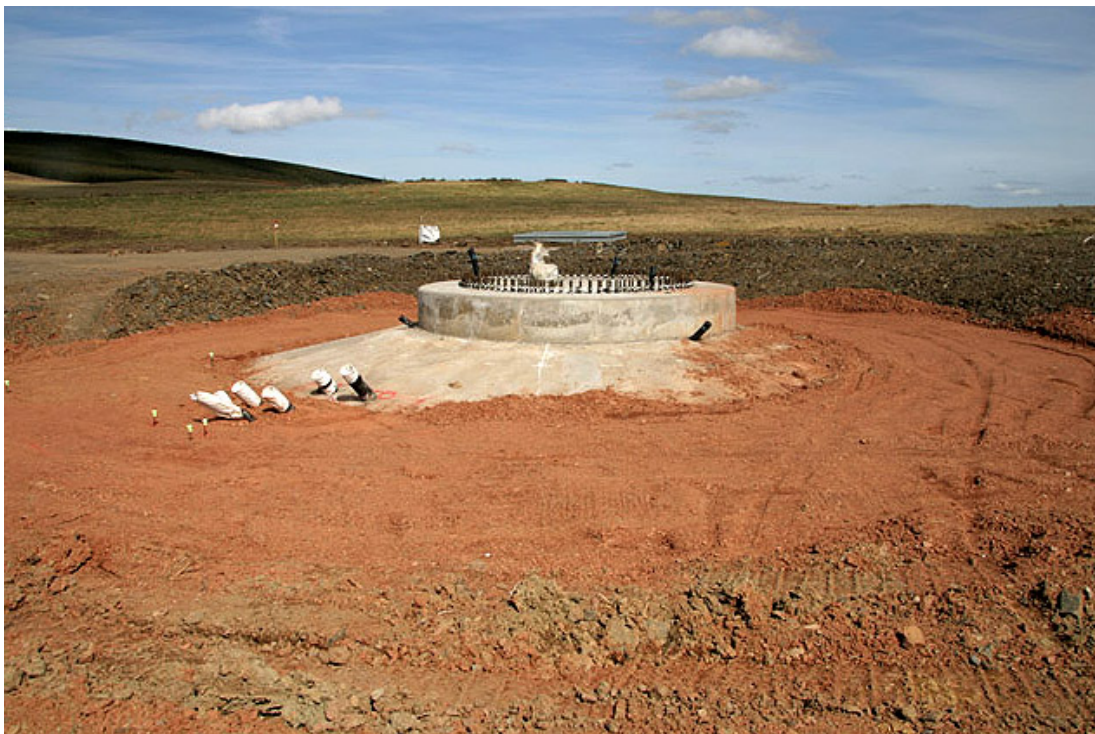
Figure 9-10: Onshore wind turbine foundation at Toddleburn wind farm, UK. [181] Licensed under CC BY-SA 2.0
