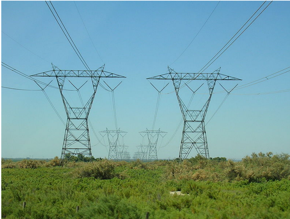
Figure 10-8: Close View of a 500kV Lines, Southern California Edison's Path 26 (Credit: RaumfahrtHauptfokus (Henristosch), Wikimedia Commons author (GNU Free Documentation License - public domain) [217])
