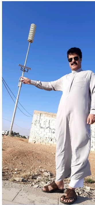
Figure 12-9: Micro solar system to supply danger horn to alert citizens during disasters
