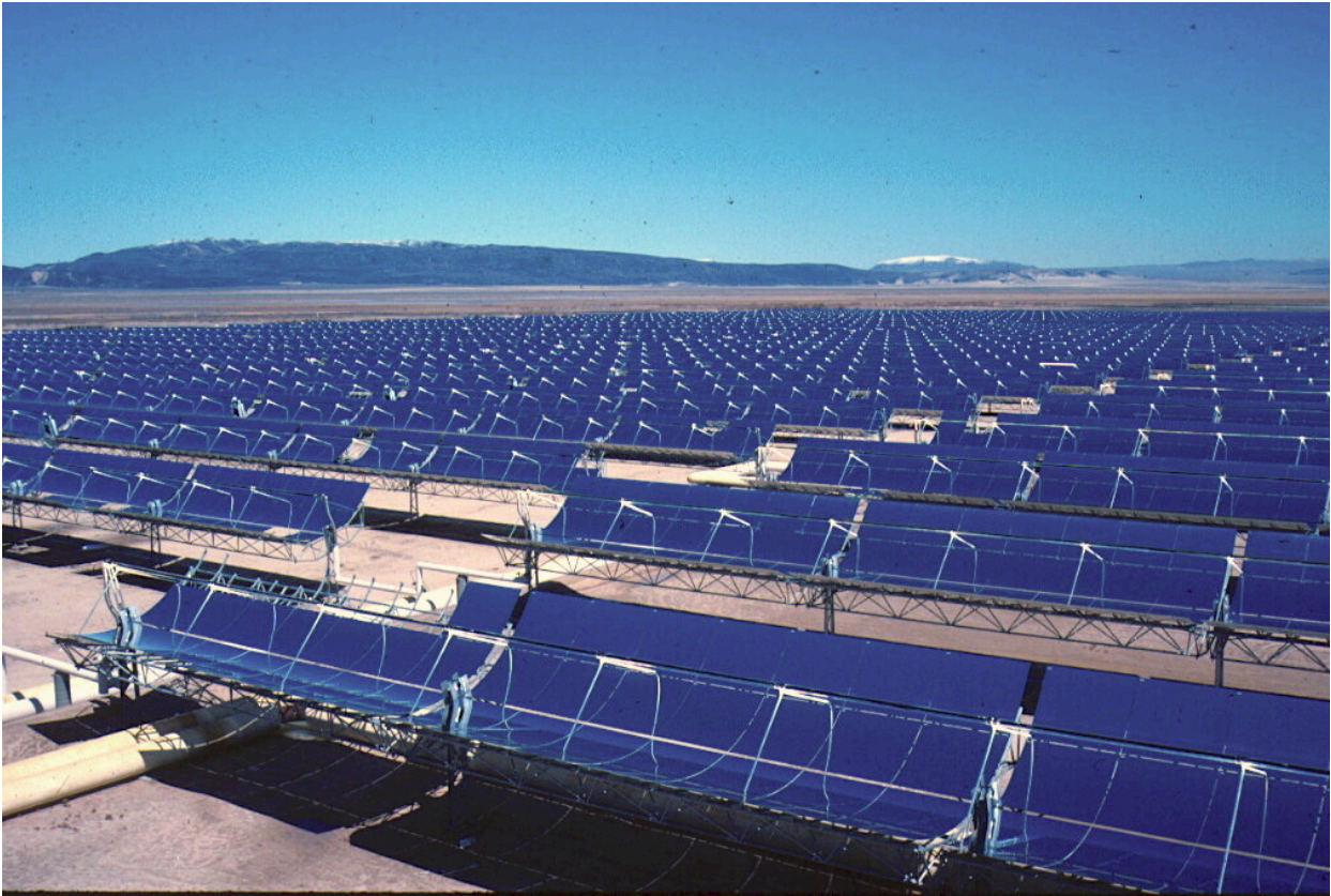
Figure 1-15: Parabolic troughs at the SEGS plant, USA. [19] License: Public Domain
