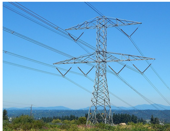
Figure 10-7: High Voltage Transmission Tower and Lines. Auburn WA, (Credit: Ron Clausen, Wikimedia Commons author (GNU Free Documentation License - public domain) [216])
