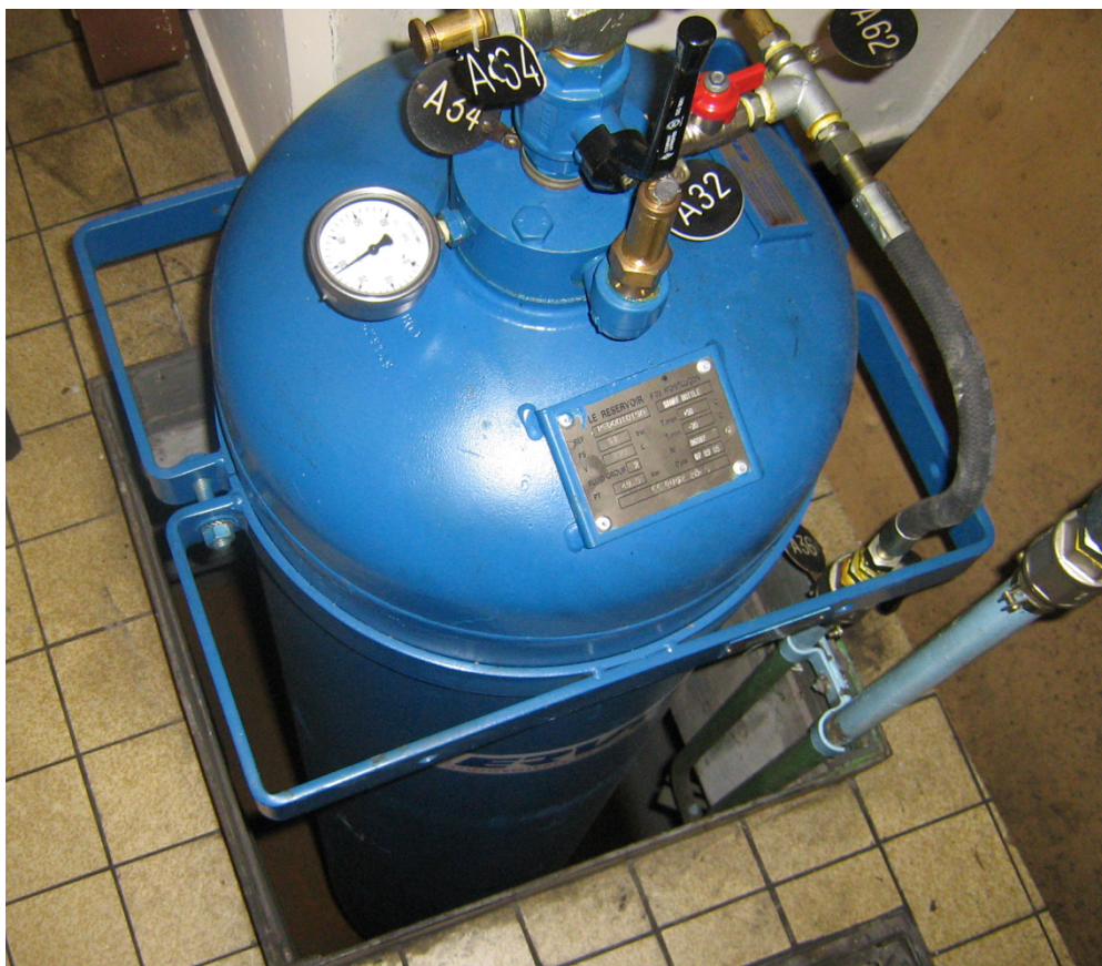
Figure 11-28: A pressurized air tank used to start a diesel generator set in Paris Metro (Credit: F1jmm under licence CC BY-SA 3.0 [410]).
