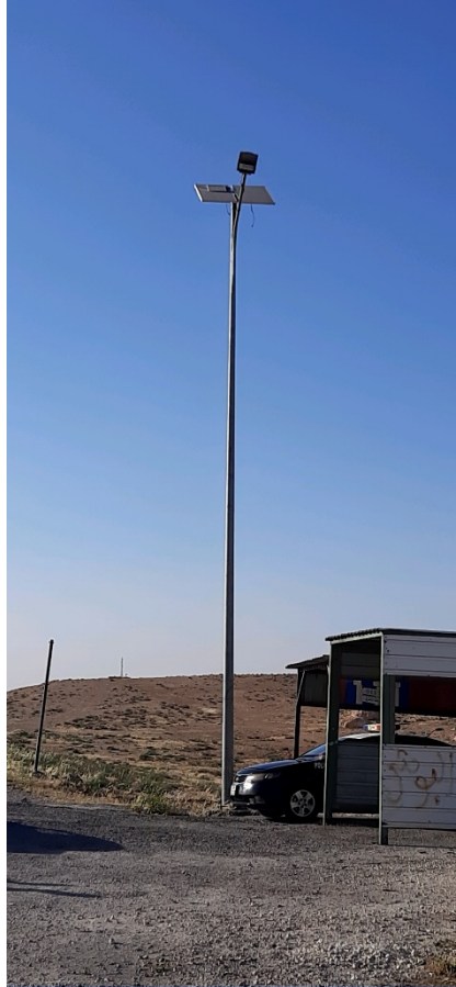
Figure 12-10: Micro stand-alone solar system for highway emergency station
